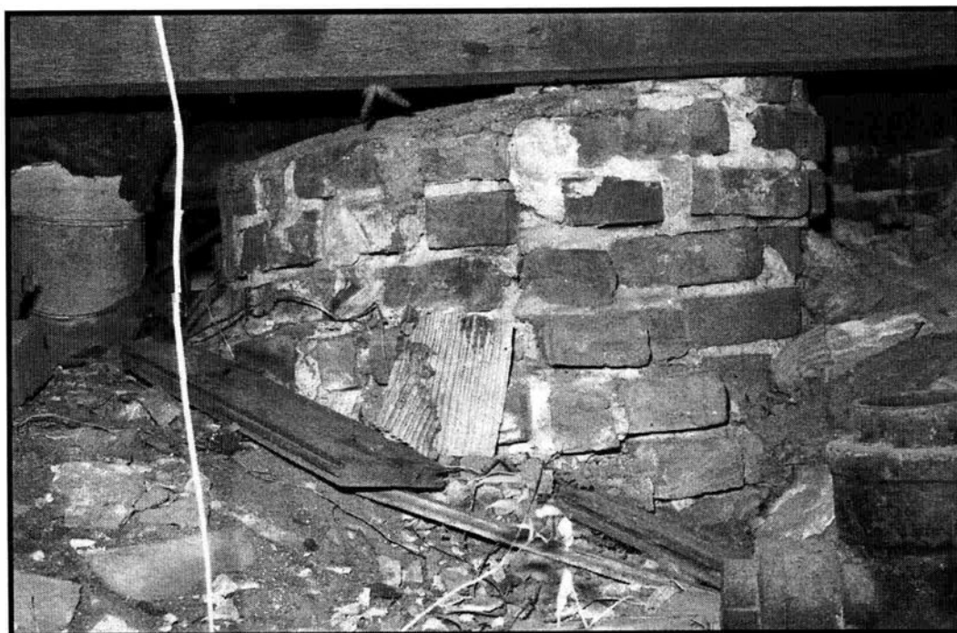
Figure 18. Cistern in Harriet Dean House crawl space.
