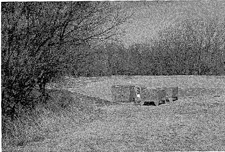
Figure 85. HVAC equipment adjacent to entry walk. [LCA, 4/96]
